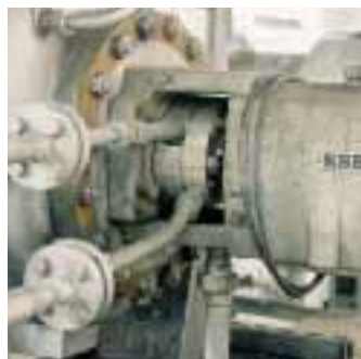
Return pump (KSB) with Burgmann tandem seal type H75S2/60-H75F2/55 according to API 682 Plan 52 for sealing C 4 hydrocarbon. Buffer medium: methanol.
