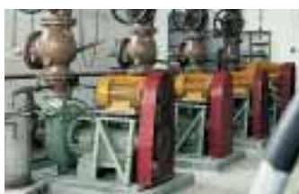
Raw sludge pumps (KSB, KRK 150–37), equipped with Burgmann type HJ977GN mechanical seals (dead-end arrangement) in the Grosslappen sewage works run by Munich Utilities. ( d_1 = 72 \text{ mm} ; p_1 = 3 \text{ bar} ; t = 15 \text{ °C} ; v_g = 6.5 \text{ m/s} ).
