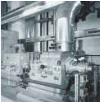
▲ Feed pump (Halberg) at Isar 1 nuclear power station with a Burgmann type SHV1/165 mechanical seal. ( p_1 = 20 bar; t_1 = 185 °C; n = 5,000 min -1 ; v_g = 47 m/s)
