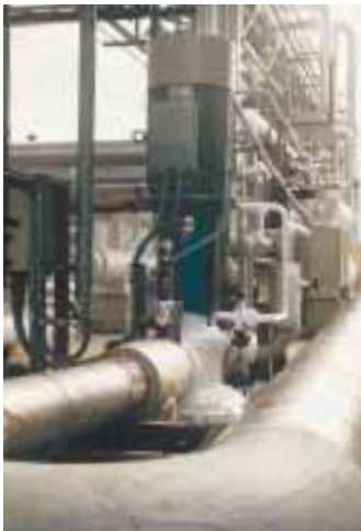
Vertical in-line pump (Worthington) for emptying an ethylene liquefied gas depot. Double sealing system with Burgmann MFLWT80F-D1/53 (API 610, Plan 53). ( p_1 = 2 bar; intake pressure = 23 bar; p_3 = 6 bar; t_1 = -103 °C; n = 3,000 min -1 ).
