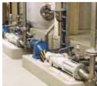
Eccentric screw pumps (Netzsch) with MG155 in paper finishing.
