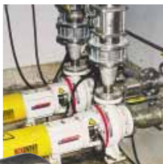
Pulp pumps (Ahlström) with LP dead-end seal
