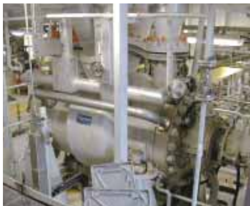
Compressor (Nuovo Pignone) on the Njord offshore platform (Norsk Hydro) with a Burgmann DGS9/130 gas seal (tandem arrangement) and a CSR to seal the bearing oil. In operation without trouble since 1998. p_1 = 26 \dots 48 bar a; n = 12,495 min -1 ; medium: natural gas.
