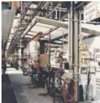
Discharge pumps (KSB, WKR-65-3) in a transfer station for propylene (C3) run by Hoechst AG, Frankfurt. They are equipped with Burgmann type H7N/H7F3 seals as tandem cartridges with TS 2000 thermosiphon system. ( p_1 = 18 bar; t = -10 \dots +40 °C; n = 2,950 min -1 ; d_1 = 38 mm.)
