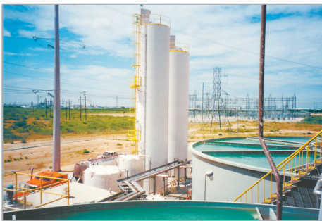
Lime / Soda Ash Storage
