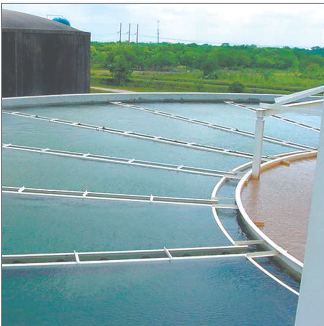
Surface Water Clarification
