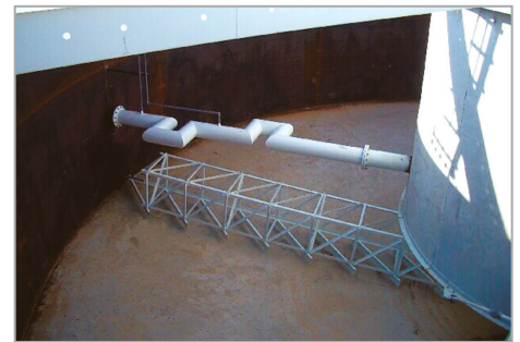
Chemical Mixing and In-line Dispersion Units
