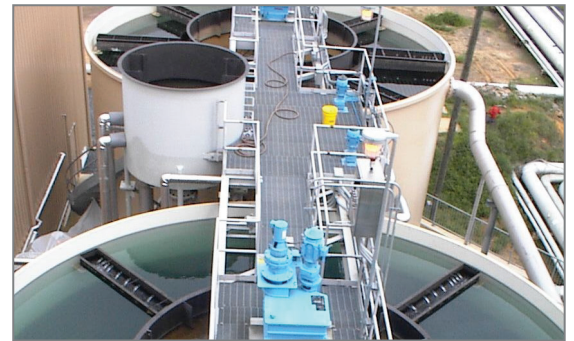
Industrial Surface Water Clarification
