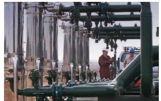
Bank of six TOPLINE housings process up to 200 cubic meters per minute
