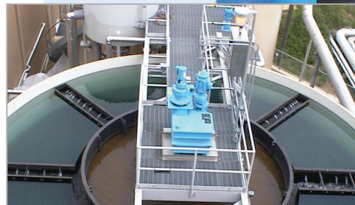
Solids Contact Clarifier
