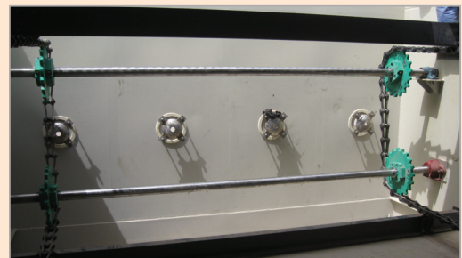
Energy Dissipating Distribution Inlets
