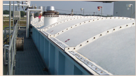
VOC Containment Cover
