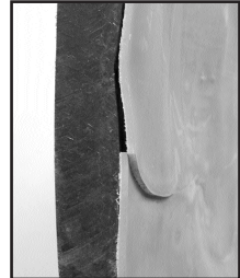
XLPE with linear liner (delamination example)
